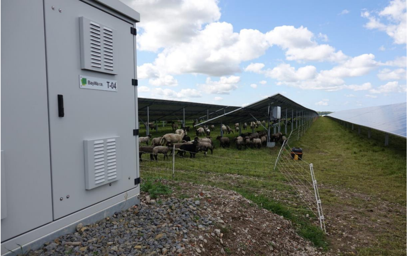
Plate 3: Typical transformer on a solar farm site
